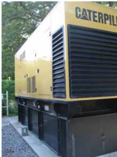
Photo 2. View of the emergency generator. The generator should be properly anchored to its foundation.
