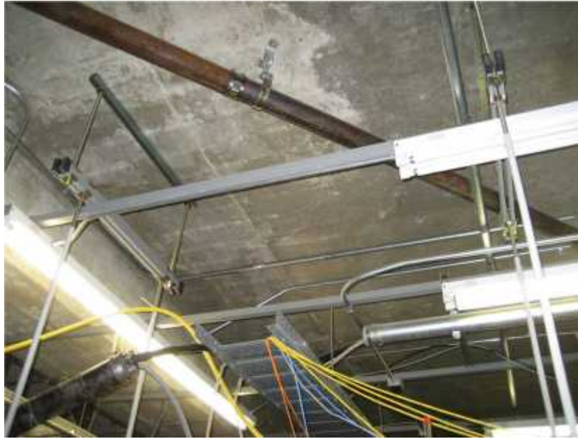
Photo 1. View of roof drain lines suspended over sensitive network equipment. Provide an alternate catchment system, such as a gutter, to prevent damage to electronic equipment.
