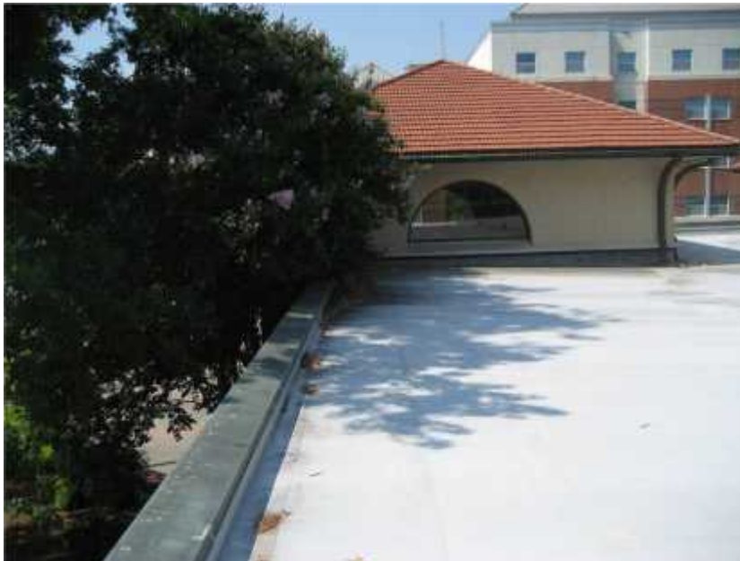
Photo 4. View of trees beginning to grow over roof. Trees should be pruned away from the facility to reduce the amount of drain clogging debris they deposit.
