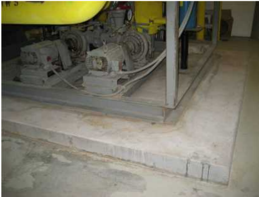
Photo 3. View of coolant/condensate pump skid not anchored to foundation. Mechanical equipment serving critical facilities should be anchored to its foundation.
