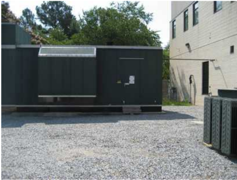
Photo 1. View of the emergency generator. Mechanical equipment supporting critical facilities should be anchored to its foundation in compliance with the building code.
