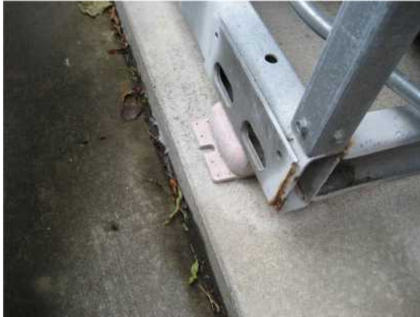
Photo 1. View of chillers at northeast corner of facility. Mechanical equipment should be properly anchored to their foundations.
