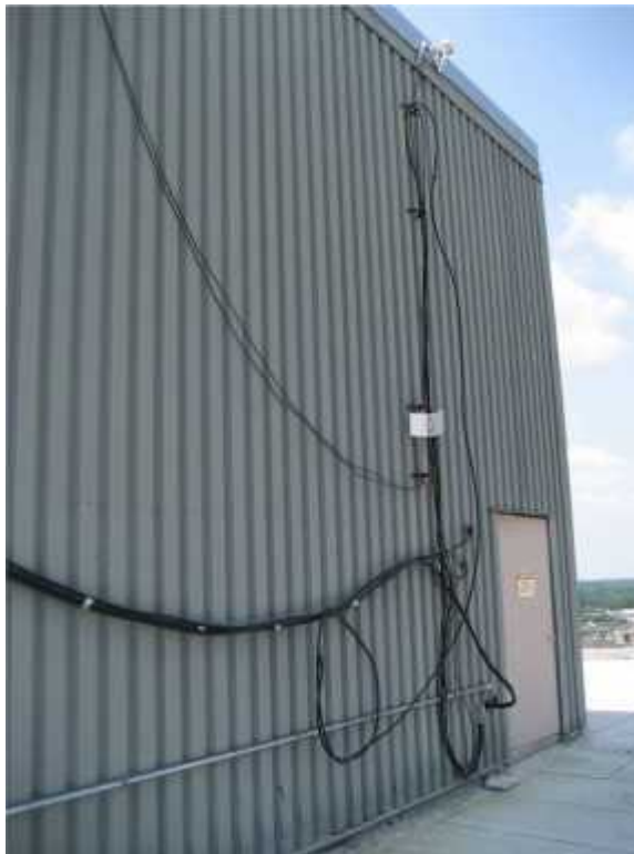
Photo 4. There are loose antennae cables attached to the outside of the mechanical penthouse. The cables should be better anchored to prevent damage in high winds.
