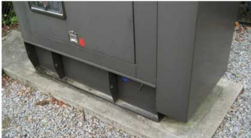
Photo 2. View of emergency generator. The generator (and the new unit in planning) should be properly anchored to its foundation.
