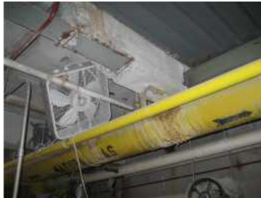
Photo 4. View of deteriorating concrete encasement in basement of steam plant. The concrete should be removed and the corrosion damage to the natural gas line repaired.
