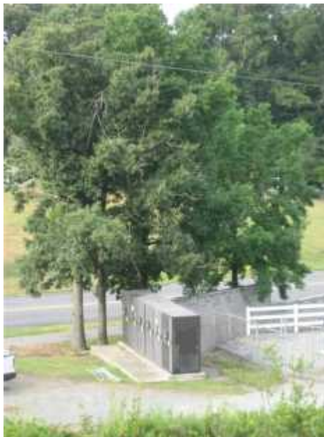
Photo 2. View of the Greenville Utility Company switchgear adjacent to peaking generators. Trees overhanging critical equipment should be routinely pruned and inspected by an arborist.
