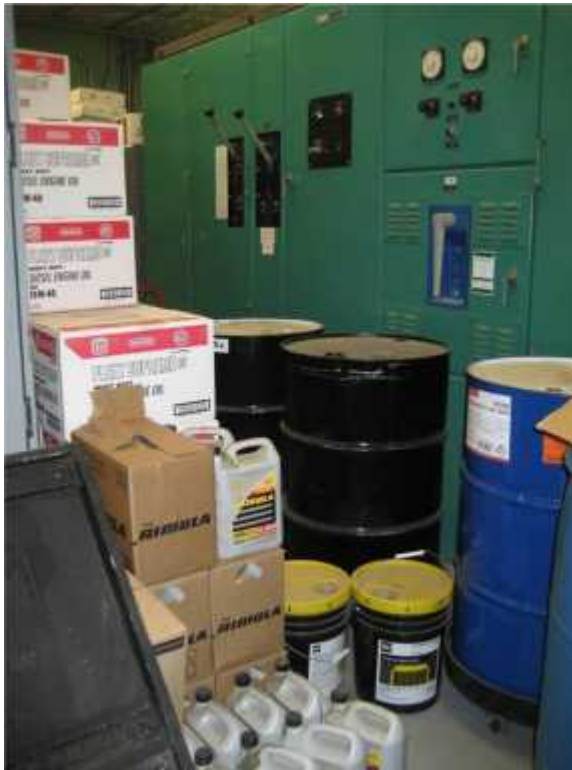
Photo 3. View of combustible materials impeding on equipment clearances. Materials should be stored in an alternate location, in accordance with code requirements.
