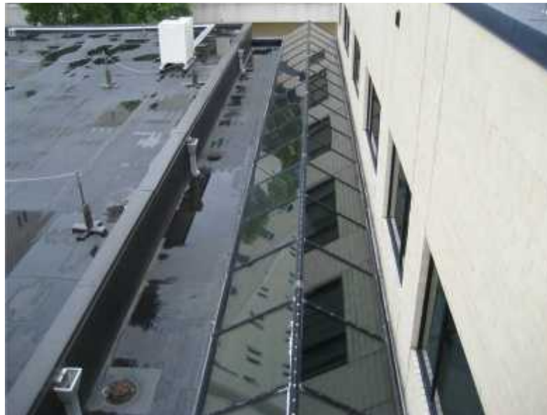
Photo 4. View of skylights over radiation therapy treatment staging area. Skylights are reported to leak during intense storms.
