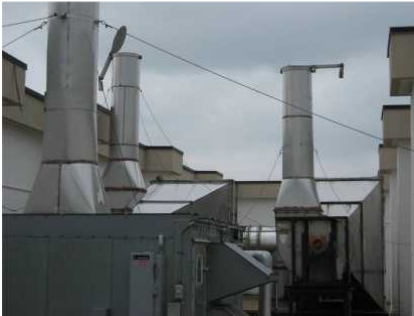
Photo 1. View of exhaust vents for BSL level 3 lab. Guide wires should be tensioned to prevent wind damage to exhaust stacks.
