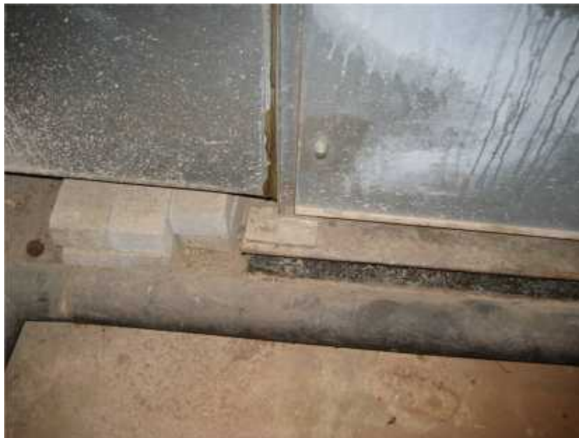
Photo 2. View of anchorage point for air handling unit for network area. The air handling unit should be anchored to its foundation.
