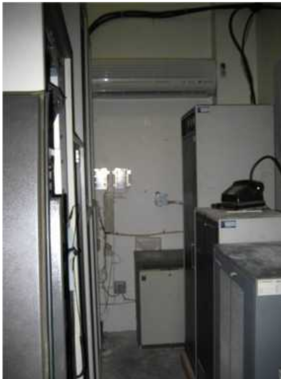
Photo 2. View of critical radio equipment in penthouse closet. The two radio rooms need smokeheads and temperature sensors.
