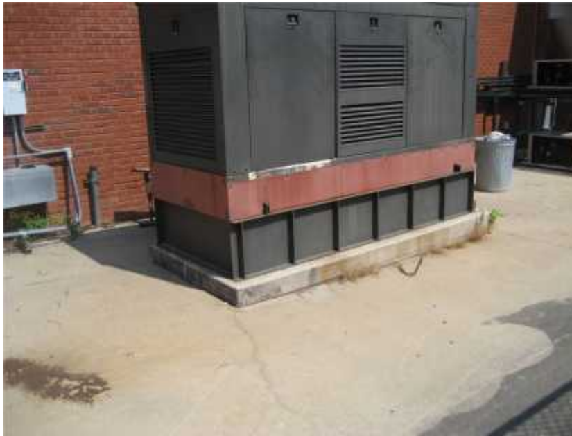
Photo 1. View of the life safety generator. The generator should be properly anchored to its foundation.
