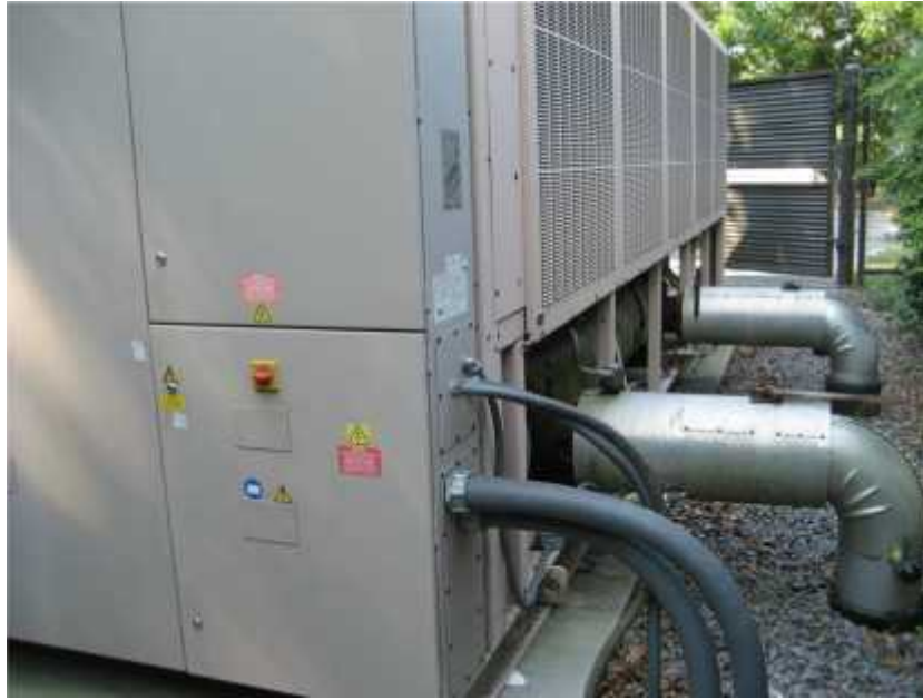
Photo 3. View of the chiller on its skid. The chiller should be properly anchored to its foundation.
