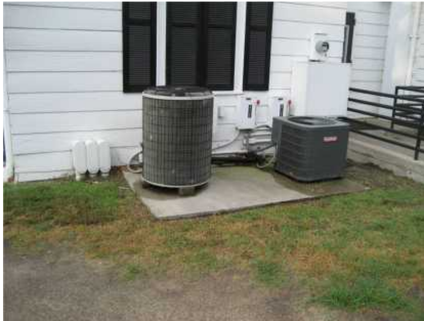
Photo 1. View of heat pumps not anchored to their foundation. Heat pumps and minisplits should be properly anchored to their foundations.
