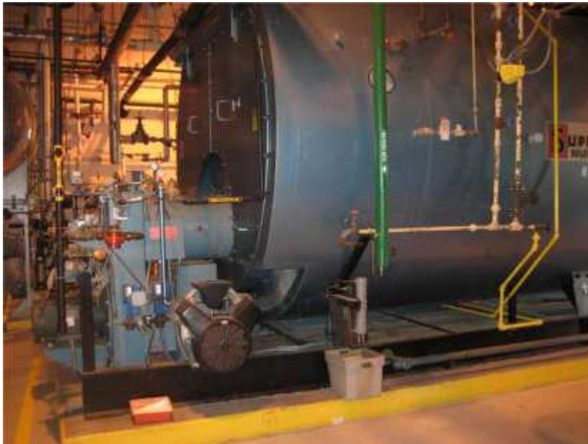
Photo 2. View of boiler. Mechanical equipment supporting critical facilities should be anchored to its foundation in compliance with the building code.
