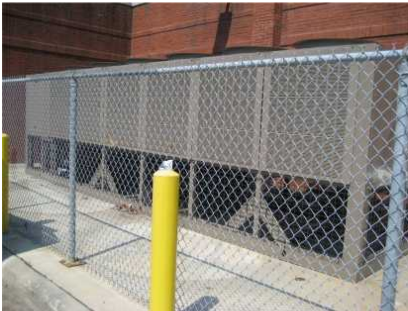
Photo 2. View of chiller unit. The chiller should be properly anchored to its foundation.
