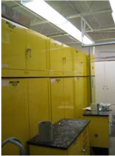
Photo 1. View of flammable storage lockers in paint shop. This area of the facility has neither fire detection or suppression systems.
