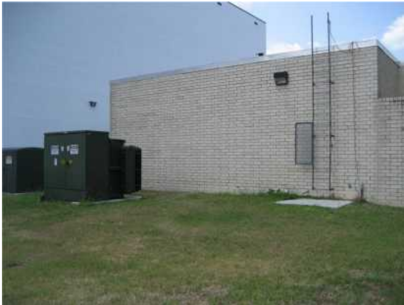
Photo 2. View of Brody emergency generator facility. The lines connecting this building to Leo Jenkins are undersized relative to available emergency power.
