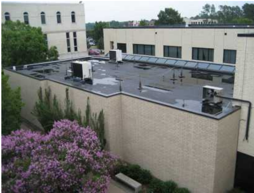
Photo 1. View of radiation treatment area of the building. The equipment inside the building and the supplemental cooling (visible on roof) do not have emergency power.
