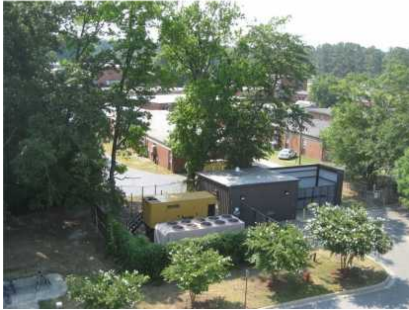
Photo 1. View of large trees overhanging emergency generator and chiller. Trees should be routinely inspected and pruned by an arborist to mitigate the potential for wind related damage.
