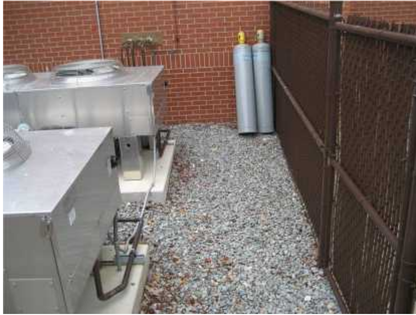
Photo 3. View of gas cylinders leaning against the southeastern exterior wall of the facility. Gas cylinders should be anchored to the wall, regardless of contents.
