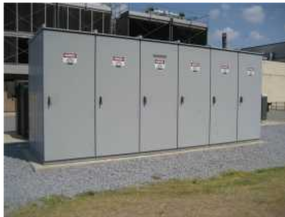
Photo 4. View of electrical switchgear susceptible to vehicle impact along the southern perimeter.
