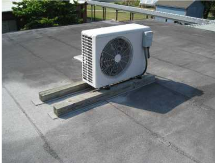
Photo 3. View of roof mounted minisplit heat pump showing supporting timbers oriented in least stable configuration. Minisplit units should be anchored to the structure.
