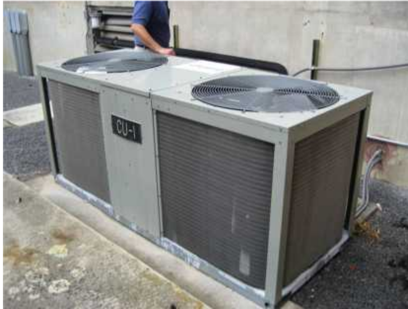
Photo 3. View of the compressor unit for the network area. The unit should be anchored to its foundation.
