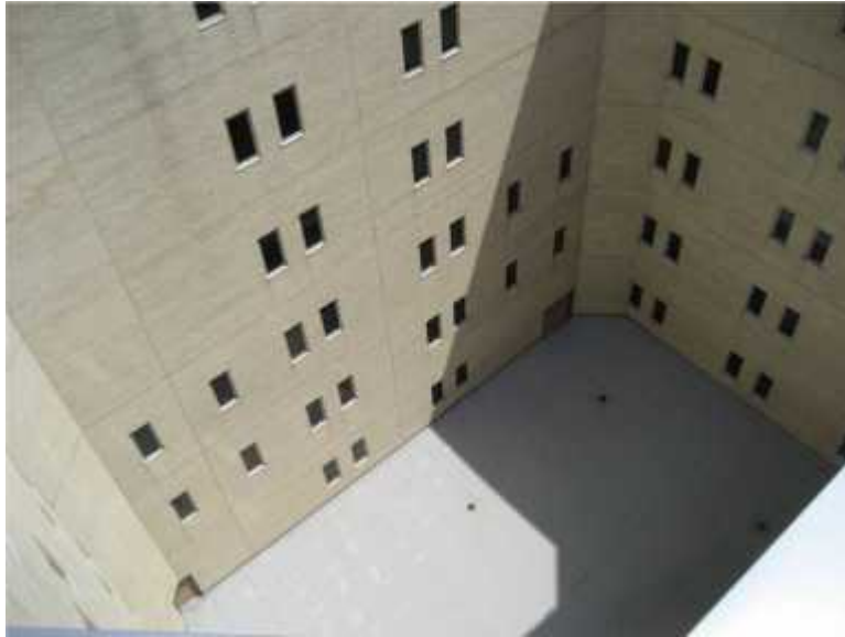
Photo 3. View of façade of interior courtyard. Several areas of the façade are reported to leak water in driving rain as a result of both improper construction and a failed remediation attempt.
