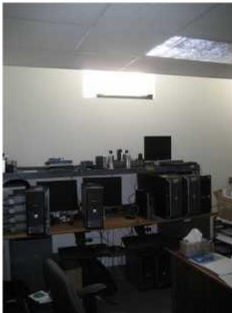
Photo 4. View of facilities management servers located in Eppes #3. If the window above the equipment were to break during a severe storm, driving rain could damage or destroy the servers.
