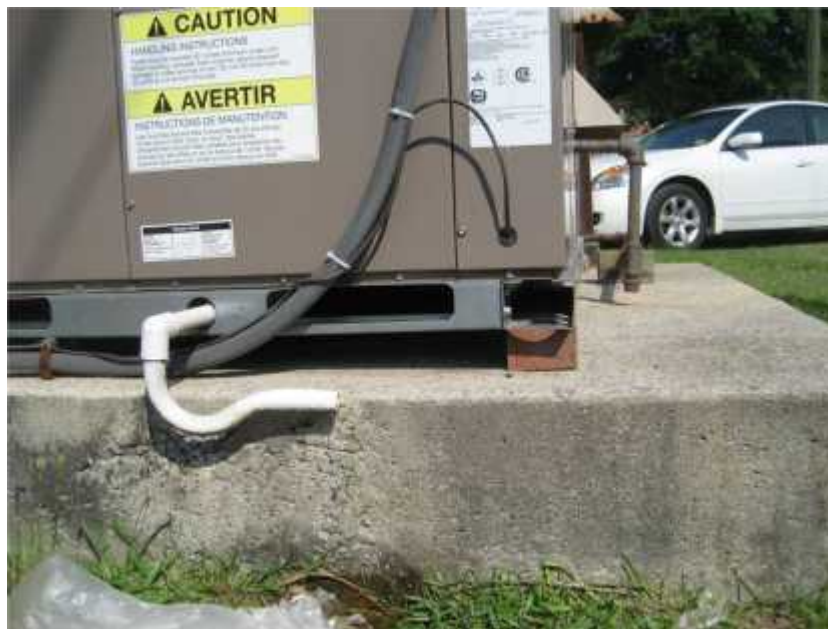
Photo 2. View of pad mounted HVAC equipment at the rear of Eppes #3. All mechanical equipment should be properly anchored to its foundation.
