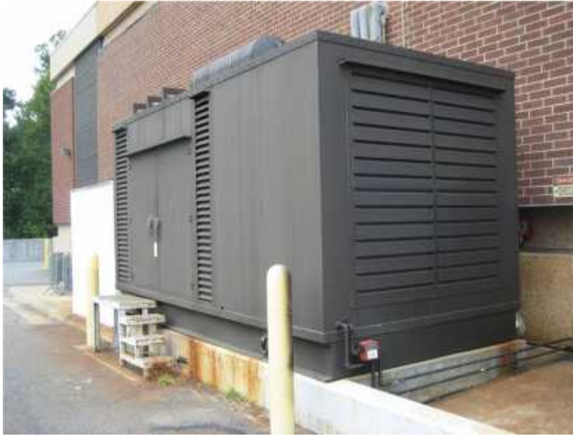
Photo 1. View of the emergency generator at the rear of the facility. Mechanical equipment should be anchored to its foundation in accordance with the building code.
