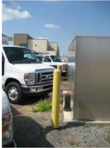
Photo 3. View of potable water backflow preventer on western perimeter subject to vehicle impact.
