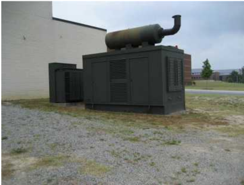
Photo 2. View of emergency generator. Mechanical equipment serving critical facilities should be anchored to its foundation.
