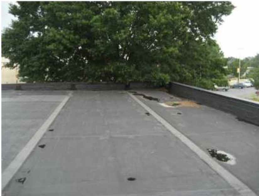
Photo 4. View of tree overhanging roof at northeast corner of facility. Trees should be pruned to reduce the likelihood of clogging roof drains.
