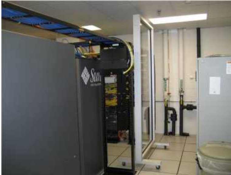
Photo 1. View of water lines in hot-site data center. Leibert unit at right uses potable water for heat rejection during power outages. Drain lines for this water are undersized and could flood the room.
