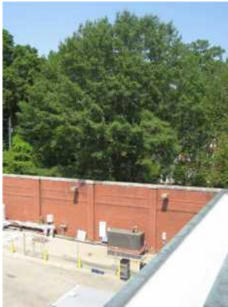
Photo 3. View of large tree adjacent to emergency generator and chiller. The tree should be regularly pruned and inspected by an arborist to decrease the likelihood of wind related damage.
