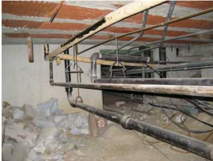
Photo 4. View of water pipes in crawlspace adjacent to network area. This area should have a water monitoring system to detect pipe leaks to prevent potential network gear damage.
